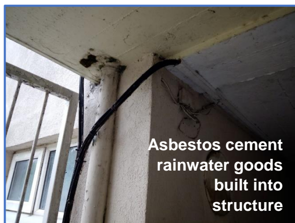
Spalling concrete in stairwell
